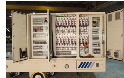
Control system on headed transporter
